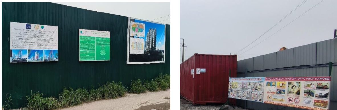
Photo 7: Informational board and warning signs installed, December 2022
